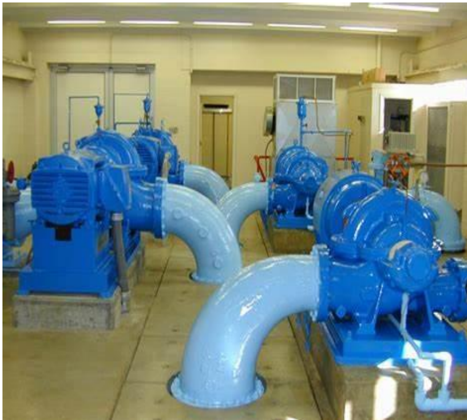
Fig.2 Installed Pumping Station
